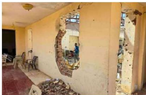
Amid ruins: Damaged interiors of a building after it was reportedly targeted by the Rapid Support Forces in El-Obeid on Monday. AFP
